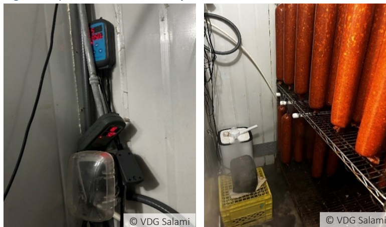
Figure 4 | Humidifier and temperature controllers
